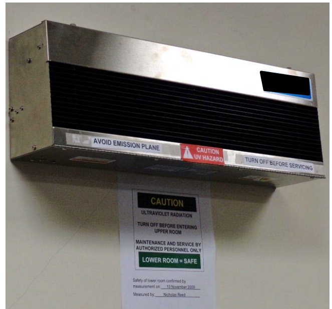
Figure 2. The UV germicidal lamp from Figure 1 is shown with more prominent safety warnings. The sign posted below states when APHC’s Nonionizing Radiation Program (NRP) evaluated the room’s UV safety and confirmed that the lower room was safe for normal work activity. It also cautions workers to turn the lamp off before climbing up to the level of the emission plane.
