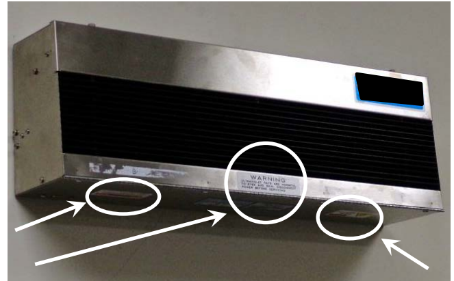
Figure 1. Upper room UV germicidal lamp. The arrows and circles highlight the lamp’s UV safety warnings, which may be overlooked even by those who install and maintain the lamps.
